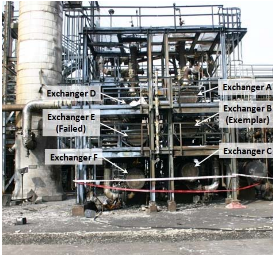
Figure 10. Six NHT Heat Exchangers in Two Banks of Three Heat Exchangers Each
